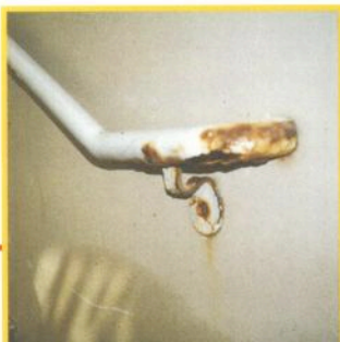
Rusted steel handrail
