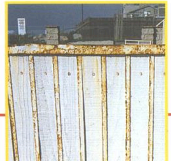
Rusted wrought iron
