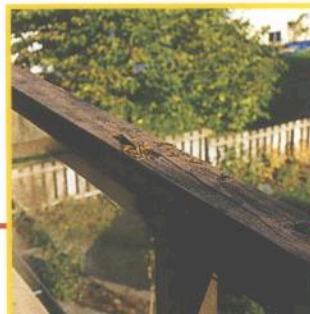
Rotting, splintering wood rail
